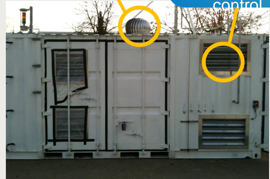
Rear side (northern) of compressor container
