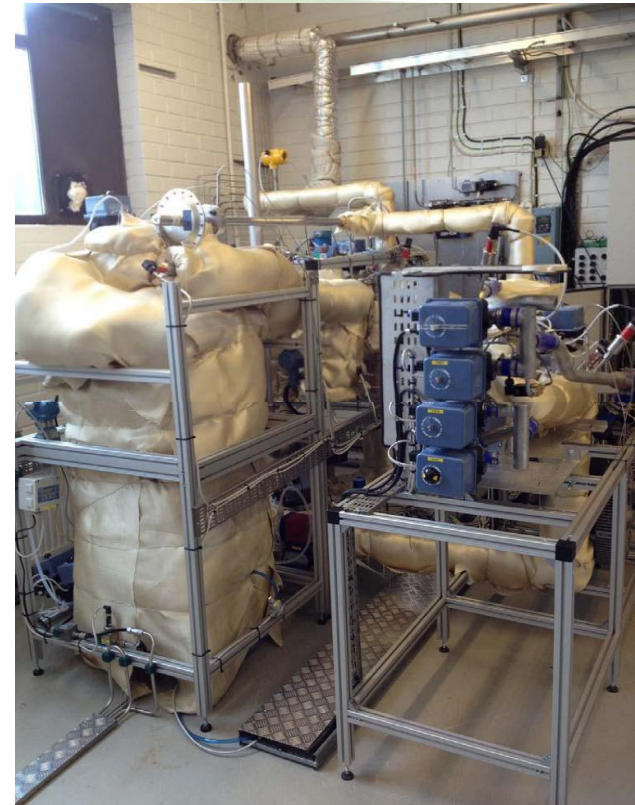
Steam ejector based recirculation test system
