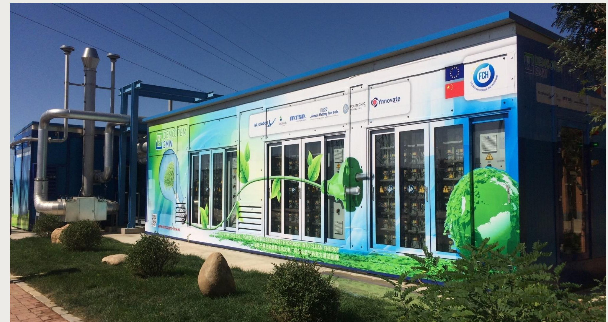
Installation at Ynnovate site, Yingkou, China
