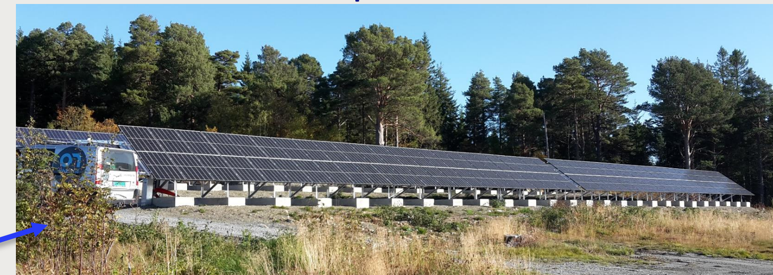
85kWp PV field
