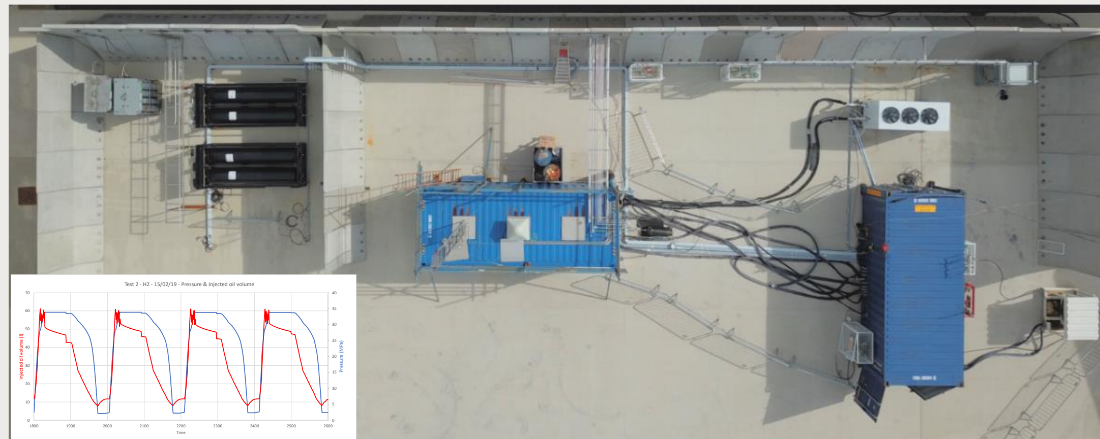
Aerial view of hydrogen test area for full scale CBM testing in closed loop
