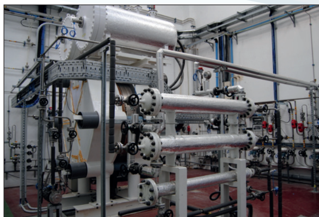
Figure: Electrolyser of IHT at FHA facilities
