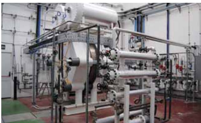
Picture of the IHT electrolyser at the FHA facilities
