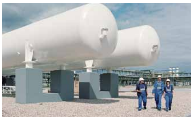
Picture: Storage vessel for liquid hydrogen, Source: Linde
