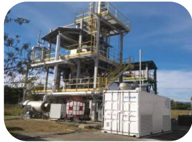
UnifHy 1MWth plant - 500kg/d
