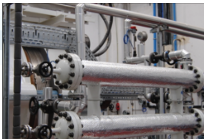
Figure: Electrolyser of IHT at FHA facilities
