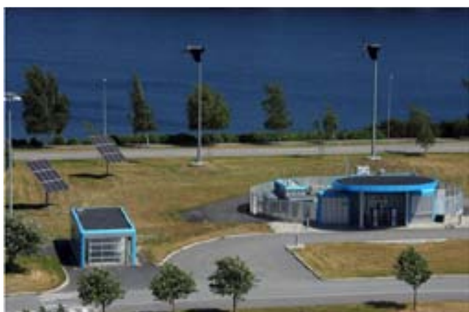
Figure 1: Statoils Energy Park at Herøya, Porsgrunn, Norway. The energy park consists of two 6 kW wind turbines and two 2.1kW solar panels and is equipped with a 70 kWh lead acid battery storage system, and water electrolysers from NEL Hydrogen (Earlier Hydrogen Technologies).
