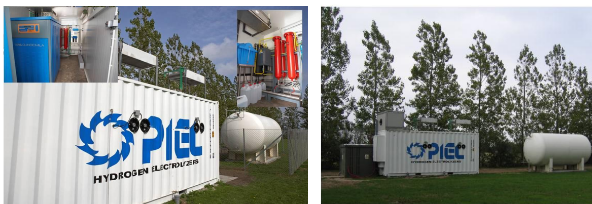
Figure 4.4. Electrolyser and storage unit.
