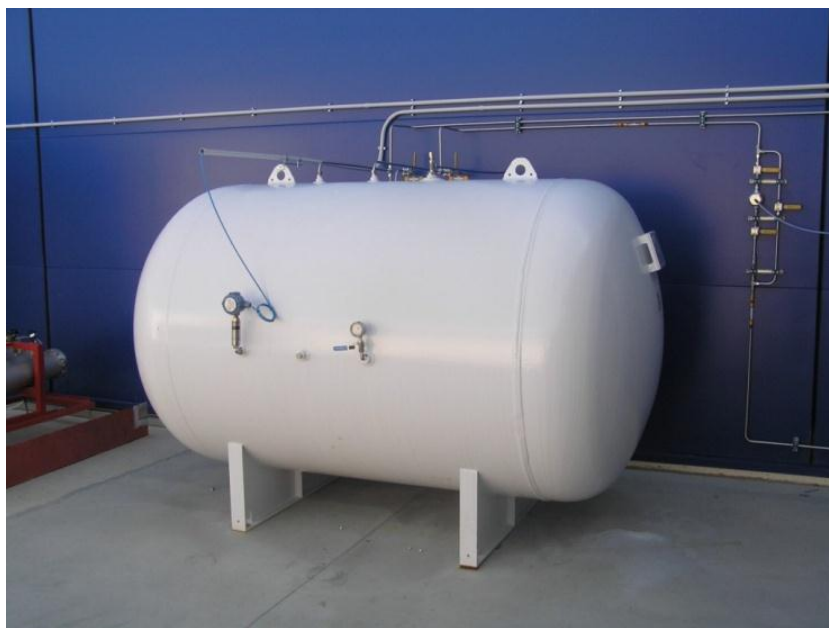
Figure 2.9. First storage stage after hydrogen production; 120 Nm 3 at 30 bar.
