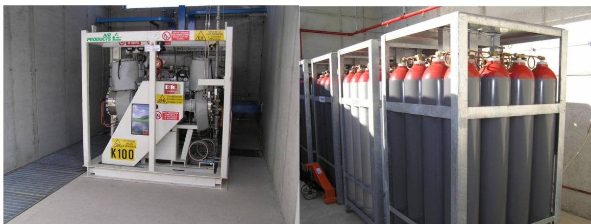
Figure 2.24. Two-stage membrane compressor (left) and cylinders groups (right) for storage in Mantova filling station.
