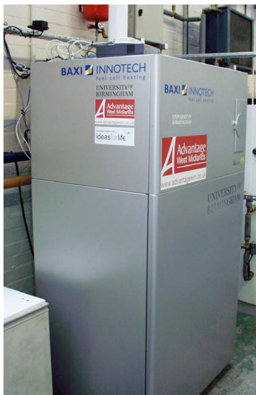
Figure 4.1. SOFC CHP system.
