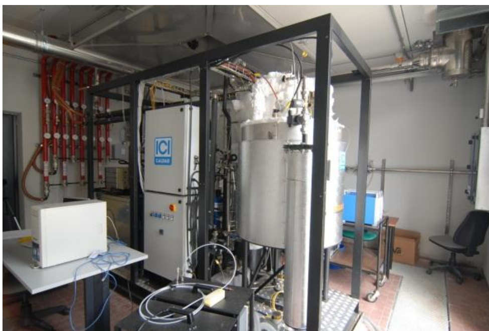
Figure 4.7. Test room with a prototype CHP plant (PEM FC system by ICI Caldaie SpA with hydrogen generated locally through a NG reformer). Hydraulic and electrical connections are on the left side, gas connection on the right. An HVAC unit and a safety ventilation system continuously refresh the room atmosphere during the tests.
