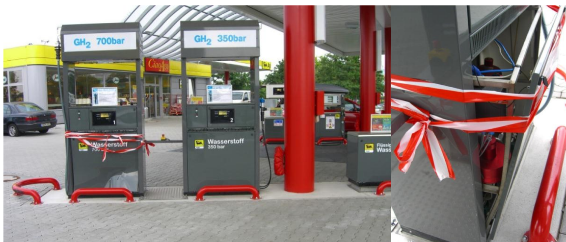
Figure 2.26. 700 bar dispenser after the accident involving
