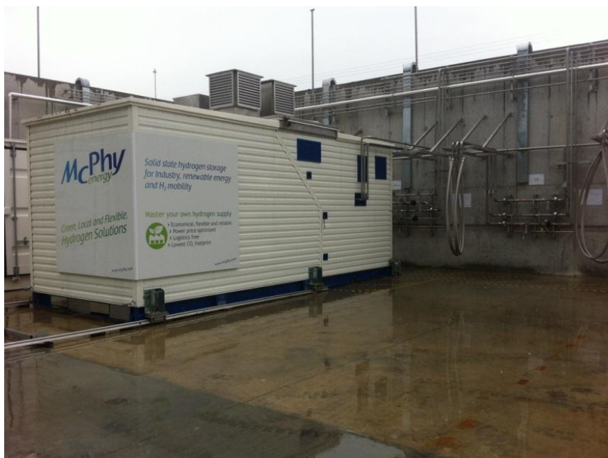
Figure 2.6. Storage system from outside.
