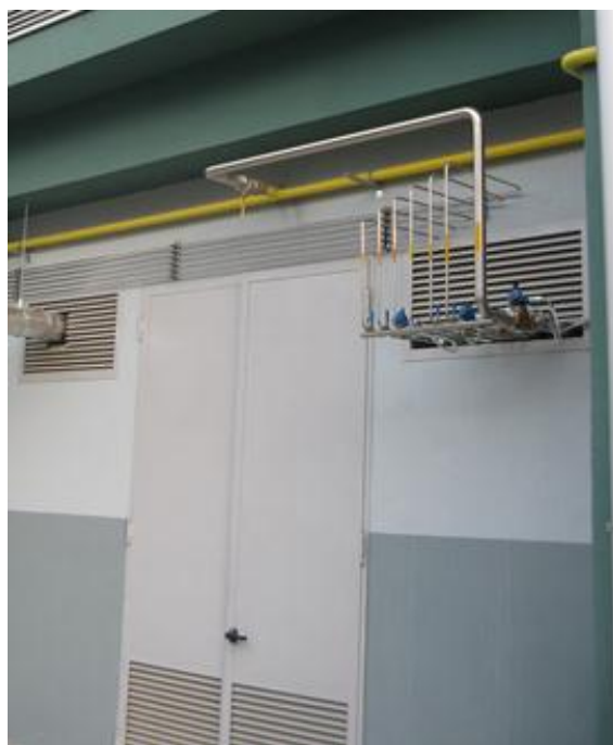
Figure 4.8. Gas lines feeding the test room from the external side, with automatically actuated valves (controlled by the gas detection system) on the right.
