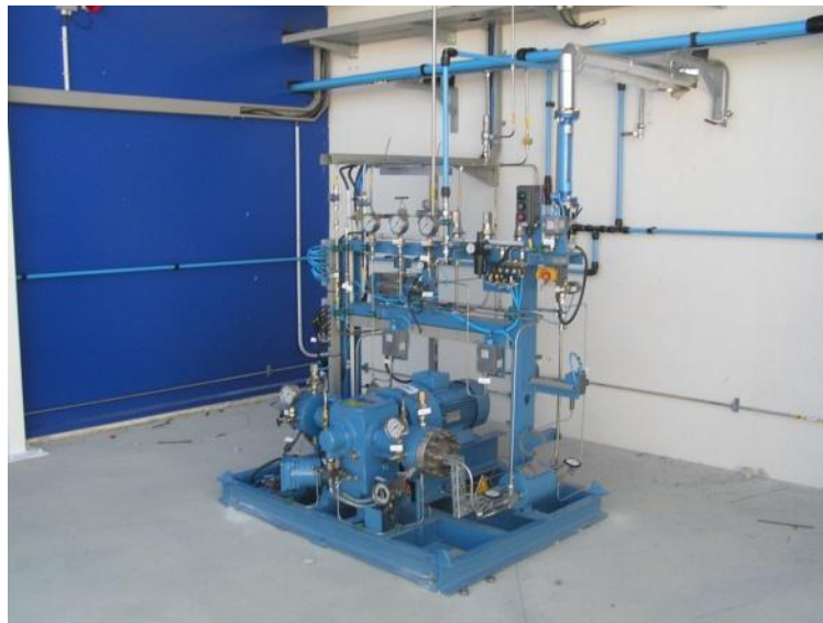
Figure 2.10. Two stages compressor, compressing hydrogen from 30 bar to 350 bar.
