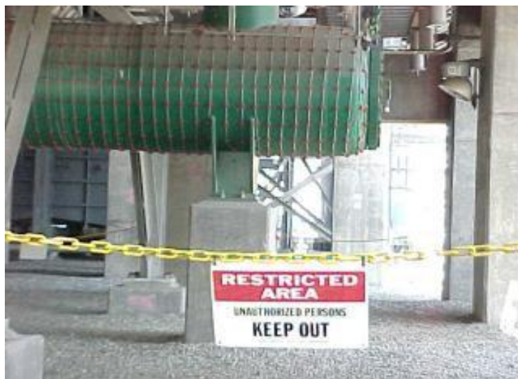
Figure 1.1. Warning signs in hazardous areas in a hydrogen plant.
