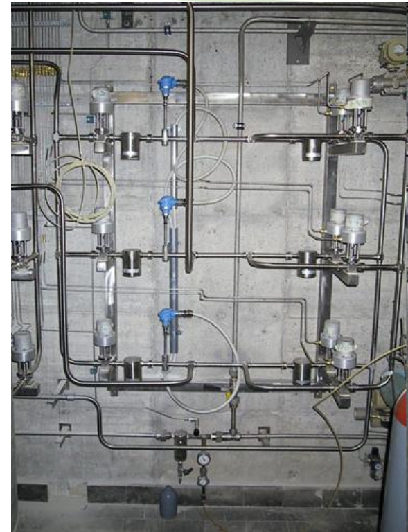
Gas purification plant from Tecnodelta
