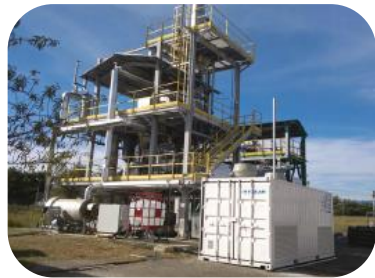
UnifHy 1MW th plant - 500kg/d
