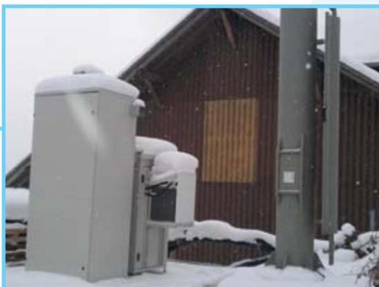
Site in Switzerland Polycom - EPS
